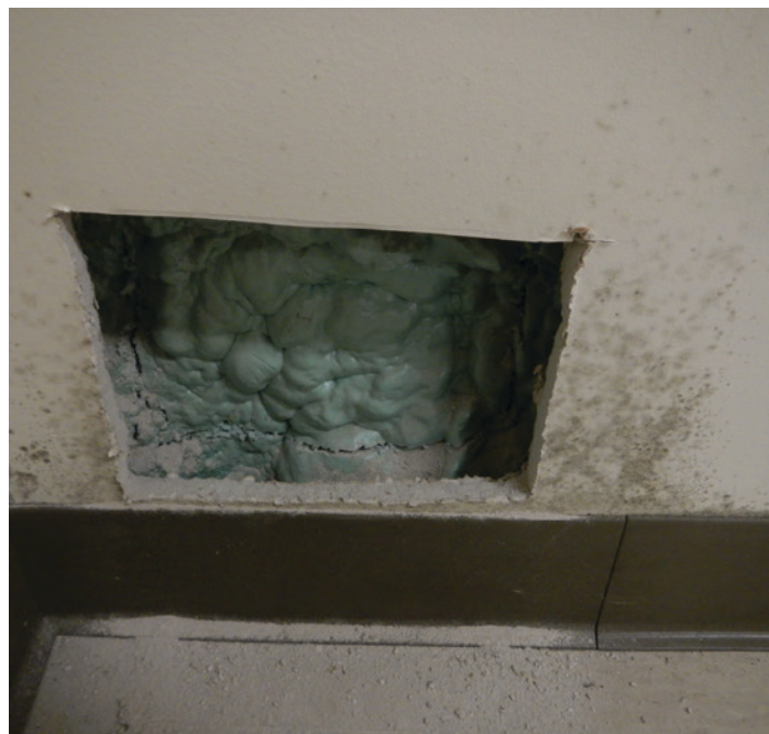
Figure 4-1 Interior Wall Showing Water Damage and Mold
