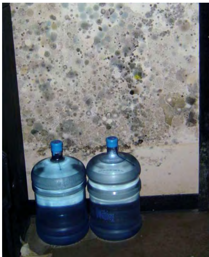
Mold growth on wall board.
